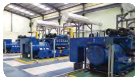
Methane Capture Plant in Kekayaan POM
